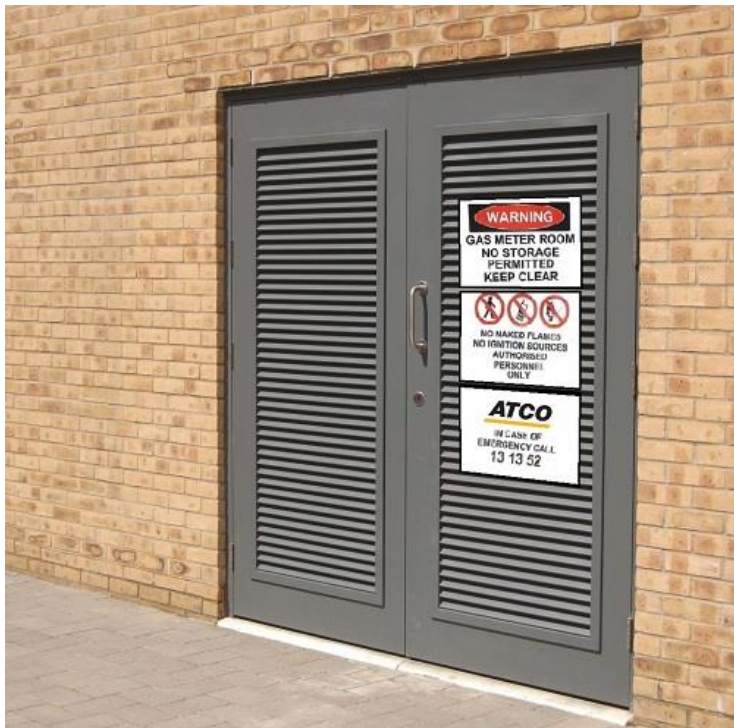
Figure 57: Meter Room – Example of Signage
