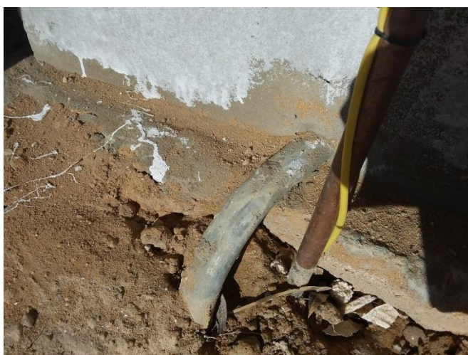
Figure 22: Non-compliant Service Separation (Less than 150 mm)
