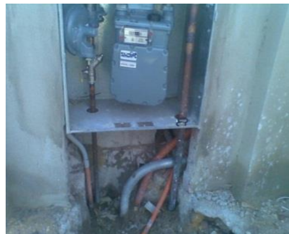
Non-conforming Installation (Other Services Installed)
